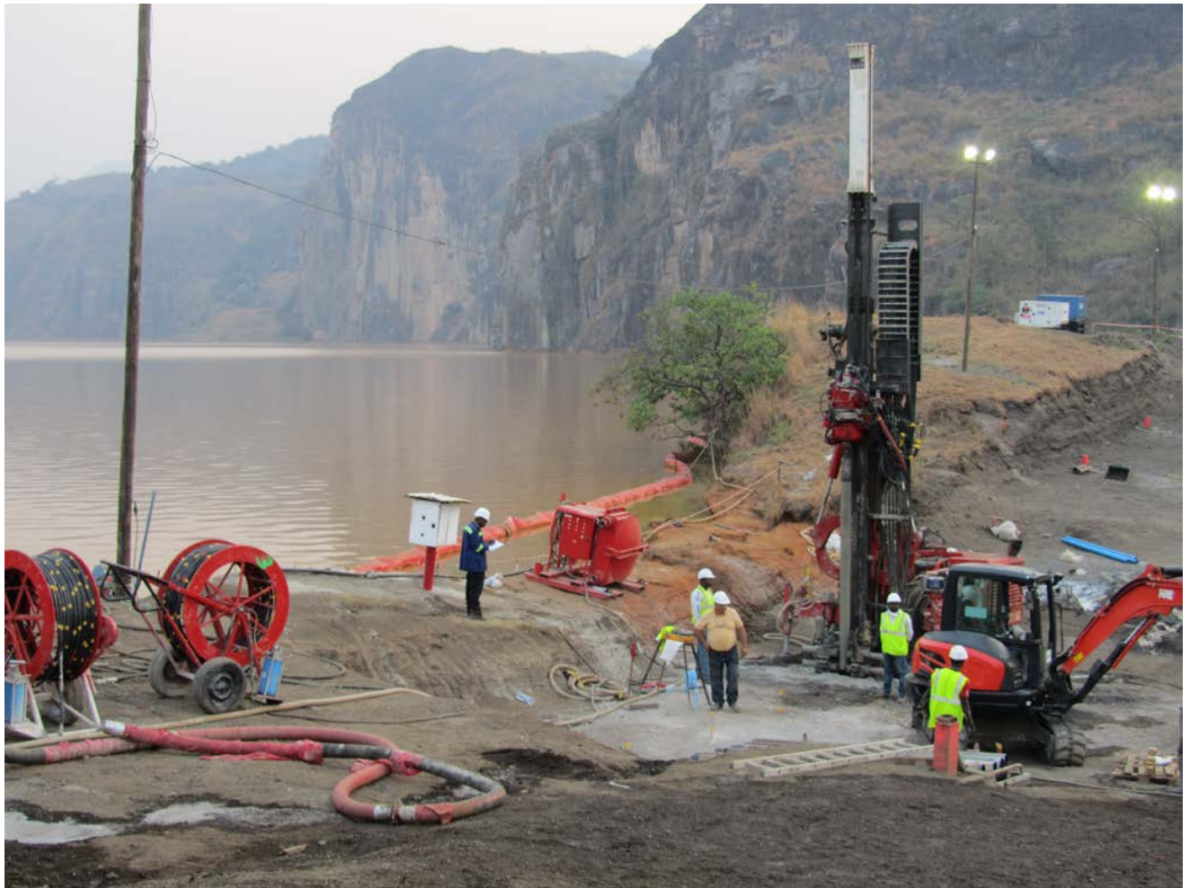
Figure 7. Operations to strengthen the weak natural dam at Lake Nyos include drilling into the dam and injecting liquid cement in order to stabilize the dam and prevent leakage of lake water through the dam. This picture was taken on 22 January 2013 and shows the drilling process across the dam.
